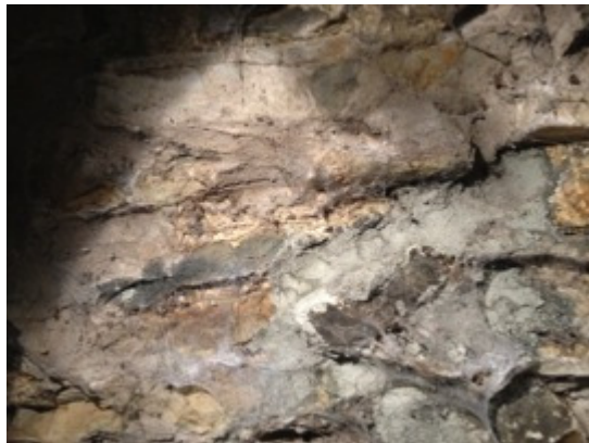
Image 2.7: The arch of the Diosig Bridge. The arch has been repointed and consequently there are only a few remaining crevices.
